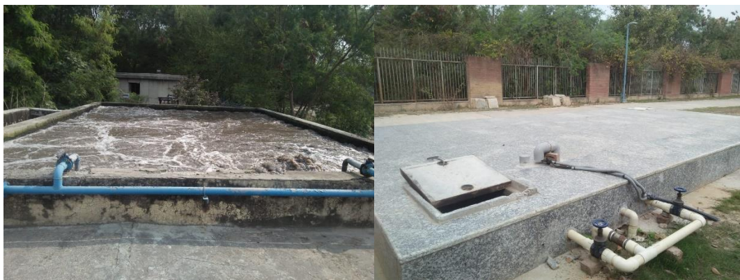
Underground Water Tank and Sewer Treatment Plant at Rajiv Gandhi Hostel for Girls, University of Delhi
