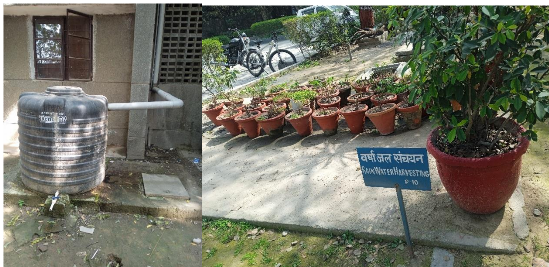
Water Tank and Rain Water Harvesting in Aravali Hostel University of Delhi South Campus
